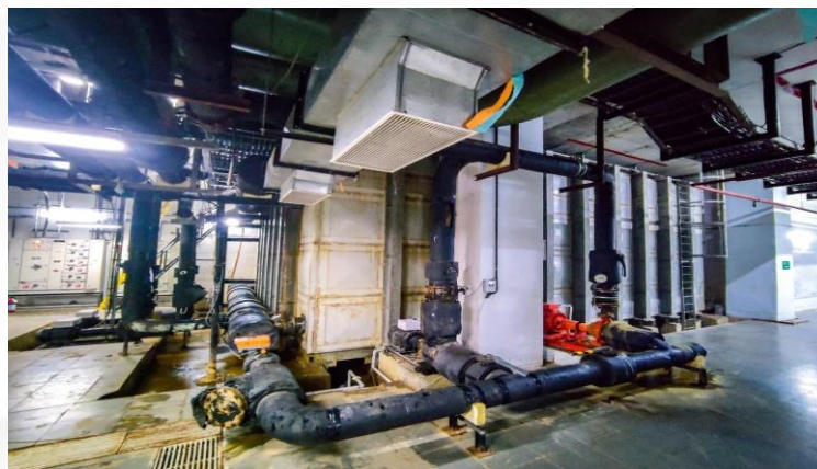
Fig. 3.2.2: Thermal Storage capacity of 3 lakh litres set up in IITMRP
